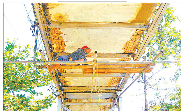
Skilled workers of Myanmar Railways led by Senior Engineer (Civil) U Than Tun of Division 5 of Toungoo and JE-II U Aung Kyaw Nyunt (Pyinmana) and party repairing the lower structure of 390 feet long overpass across Pyinmana Station Yard of Myanmar Railways on 19 December.— MYANMA ALINN
