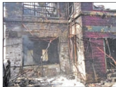
A view of a building damaged by a suicide bombing is seen in Nigeria's northern city of Kano on 22 Dec, 2012.
