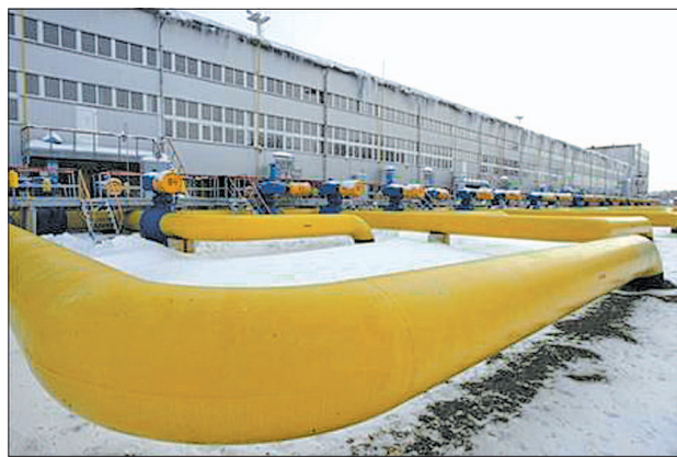
Pipes are seen at a gas compressor station in the village of Boyarka, outside Kiev, on 19 Dec, 2012.
