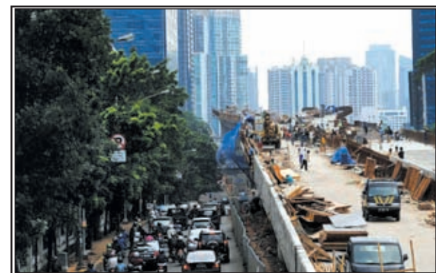
Vehicles drive past the construction site of a viaduct bridge in Jakarta, Indonesia, on 20 Dec, 2012. Indonesia's economic growth is expected to reach 6.6 percent in 2013, according to an official of Asian Development Bank.—XINHUA
