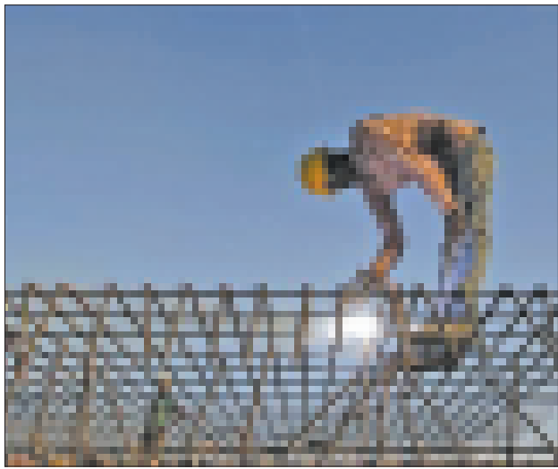
A worker welds iron rods at the construction site of a commercial complex in Ahmedabad on 29 Nov, 2012.—REUTERS
