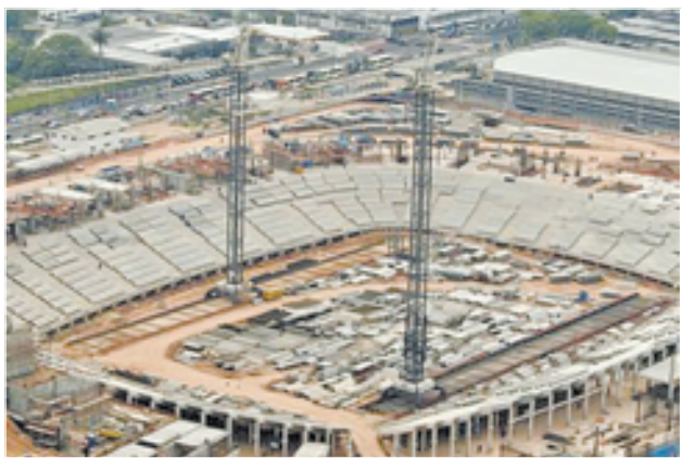
An aerial view shows the construction site of the Arena da Amazonia, or Vivaldo Lima Stadium, as it is rebuilt to host the 2014 World Cup, in Manaus on 8 Oct, 2012.—REUTERS
