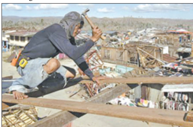
A man repairs the roof of his house damaged in the coastal town of Banganga that was devastated at the height of last Tuesday's Typhoon Bopha in Davao Oriental in southern Philippines on 11 December, 2012.
