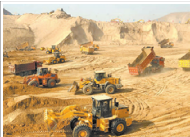
Construction vehicles work at a hilly region in Lanzhou, capital of northwest China’s Gansu Province, on 10 Dec, 2012. A project of land development has been under construction here since this October as the city planned to remove some of its barren hills to provide land of 25 square kilometres in half a year for city development.
