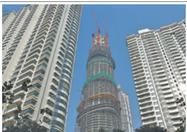
Photo taken on 8 Dec, 2012 shows the Shanghai Tower (C), a skyscraper under construction, in Pudong, east China's Shanghai Municipality. The Shanghai Tower is expected to reach 632 metres in height and start service in 2015.
