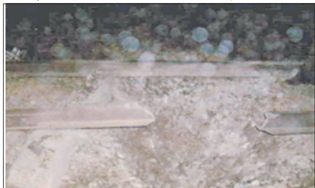
Damage of rail tracks in blast of mine planted by KIA (Kachin) group one mile south of Nanma Station.—MNA
