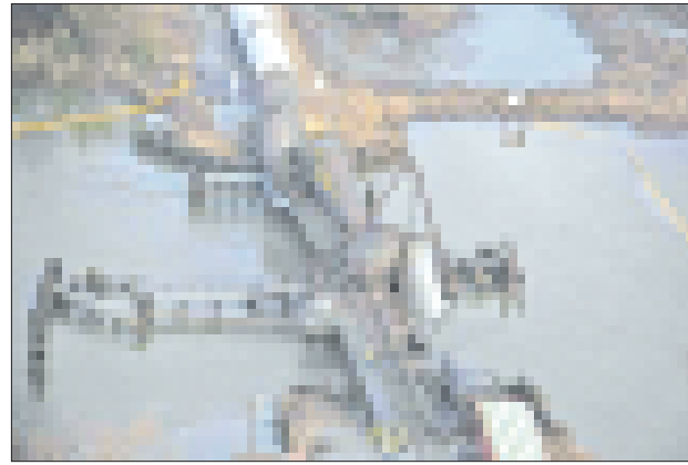
Derailed freight train cars sit semi-submerged in the waters of Mantua Creek after a train crash in Paulsboro, New Jersey on 30 Nov, 2012. A rail bridge collapsed on Friday over a creek in southern New Jersey, causing a Conrail freight train to derail and spill hazardous chemicals into the air and water, authorities said.
