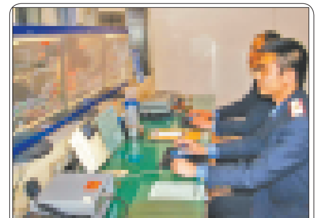
Technicians monitor the indicating maps of signals at the signal mechanical room of the Baotou East Station of the Baotou electricity section of the Hohhot Railway Bureau in Baotou, north China's Inner Mongolia Autonomous Region, Nov. 29, 2012. Facing the low temperatures, strong winds and snowfalls since winter, the Hohhot Railway Bureau has organized all its departments to guarantee the rail transport in winter, including activities like strengthening vehicle scheduling and security inspection during on-site operations.
