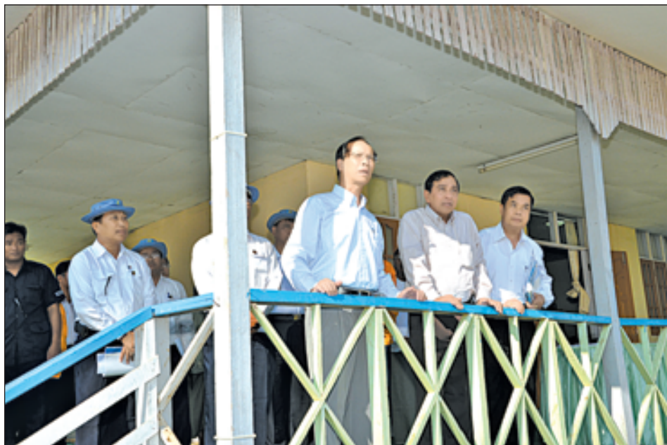
Vice-President Dr Sai Mauk Kham views damages of Ayeyawady Bridge (Yadana Theingha).—MNA
