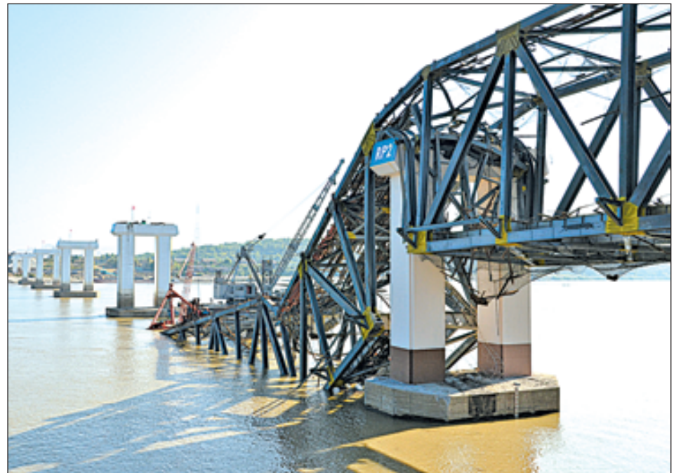
Photo shows damaged frame of Ayeyawady Bridge (Yadana Theingha) in recent earthquake.—MNA
