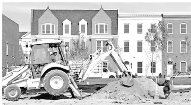
Workers prepare a new housing lot at a construction site in Alexandria, Virginia on 17 Oct, 2012. REUTERS
