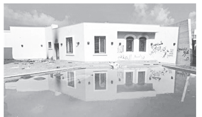
An exterior view of the US consulate, which was attacked and set on fire by gunmen, in Benghazi on 12 Sept, 2012.—REUTERS
