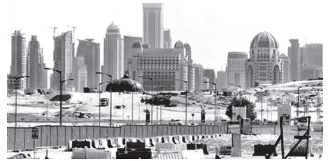
Construction cranes and bulldozers operate at a real estate construction site being built by Qatar's Lucille properties in Doha on 25 September, 2012.—REUTERS
