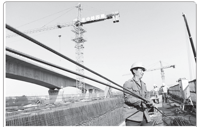
A worker works at the construction site of the Anhui section of Hefei-Fuzhou Railway in Hefei, capital of east China's Anhui Province, on 29 Sept, 2012.
