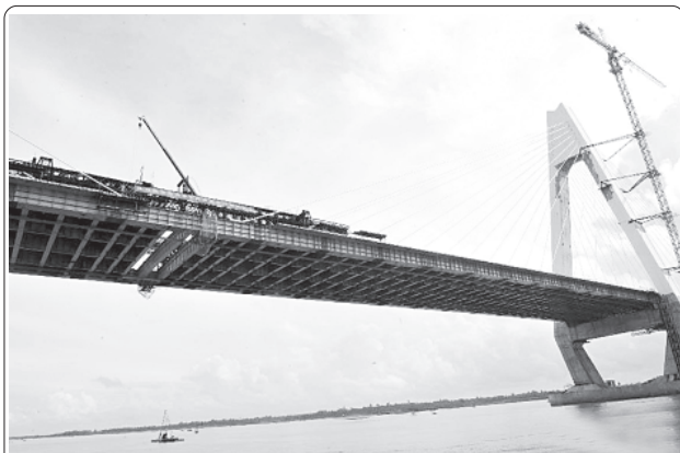
The Qinglan bridge under construction is seen in Wenchang, south China's Hainan Province, 25 Sept, 2012. The 1828-meter-long Qinglan bridge is the second cross-sea bridge of Hainan Province with an investment of 595 million yuan (94.4 million US dollars).—XINHUA
