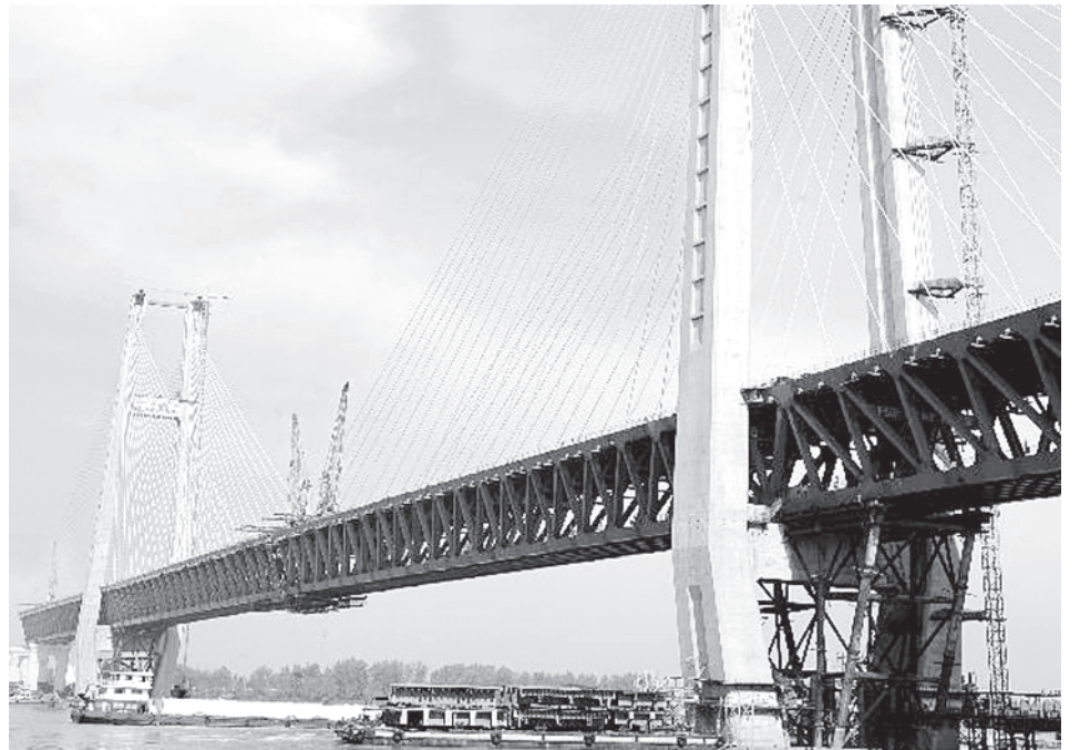
The two parts of a road-rail bridge are seen joined together over the Yangtze River in Huanggang, central China's Hubei Province, on 16 Sept, 2012. The joining work of the Huanggang Yangtze River bridge, the 6th road-rail bridge over the river, is finished on Sunday in Huanggang, Hubei Province. — XINHUA
