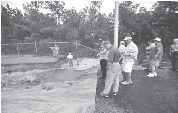
St Tammany officials inspect lock two of the Pearl River Navigational Canal after Hurricane Isaac in Bush, Louisiana, on 1 September, 2012.—REUTERS
