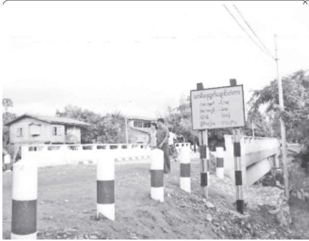
The State has constructed two-way reinforced concrete bridge at the exit of Mohnyin on Shwebo-Myitkyina Road at a cost of K 150 million recently as the old was damaged in torrential rains last year. NLM 001
