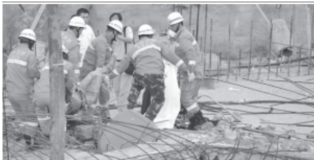
Rescuers remove an injured person at the accident site after a carpet factory building under construction collapsed in Yulin City, northwest China's Shaanxi Province, on 22 Aug, 2012.— XINHUA
