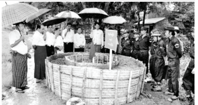
FLOODS PREVENTION TAKEN: A demonstration on prevention against floods in 2012 monsoon was held No 3 outpost of Ayeyawady-Hinthada embankment 25/1 (Hsantan) in Zalun Township of Hinthada District on 7 August. Staff Officer U Aung Swe of Township Irrigation Department performs demonstration on protection of embankment.—MYANMA ALIN
