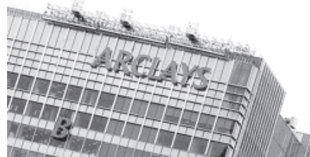
The letter "B" of the signage on the Barclays headquarters in Canary Wharf is hoisted up the side of the building in London on 20 July, 2012. — REUTERS
