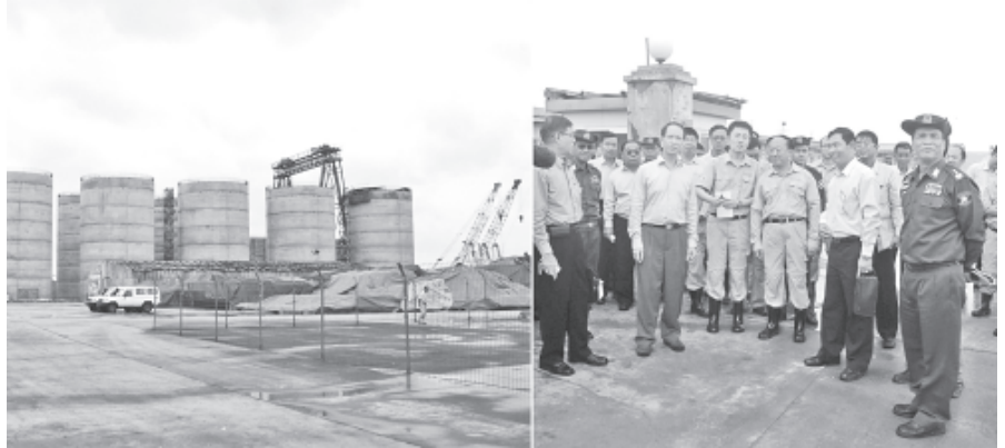
Vice-President Dr Sai Mauk Kham inspects progress in laying of Myanmar-China oil and natural gas pipelines project.—MNA
