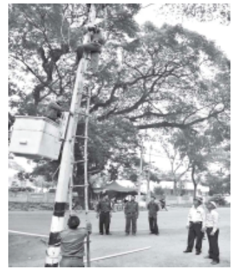
DIGITAL METER INSTALLED: Managing Director U Myint Aung of Electricity Supply Enterprise inspects installation of digital meter on Yangon-Mandalay Highway by electricians of the enterprise in Lewe Township on 21 July.— KYEMON
