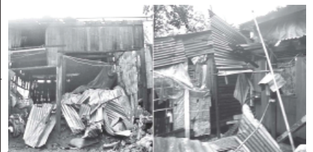
Houses collapse in strong wind-hit area of Thingangyun Township on 21 July.
