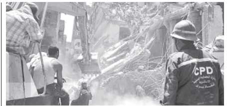
Rescue workers use heavy equipment to remove rubble and look for survivors buried under debris of damaged buildings following the collapse of an 11-story building under construction onto three adjacent buildings that killed at least 10 people in the Gomrouk neighbourhood of Alexandria, Egypt, on 15 July, 2012.—INTERNET
