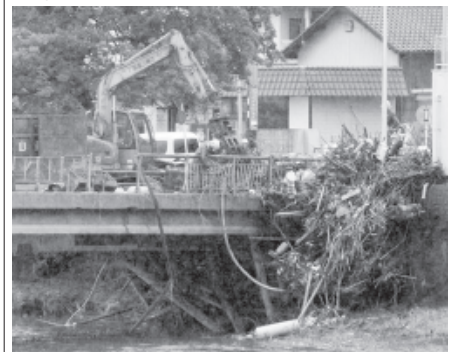
Workers remove debris from the railing of a bridge in Kumamoto prefecture, on Japan's southern island of Kyushu, on 13 July. Evacuation orders had been issued to about 240,000 people in the north of Kyushu where more rivers burst their banks, public broadcaster NHK and Jiji Press news agency reported, compiling figures from various authorities. —INTERNET
