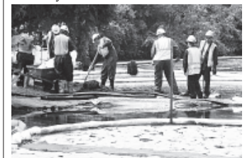
In this 30 July, 2010 file photo, crews clean up oil, from a ruptured pipeline, owned by Enbridge Inc, near booms and absorbent materials where Talmadge Creek meets the Kalamazoo River as in Marshall Township, Mich.—INTERNET
