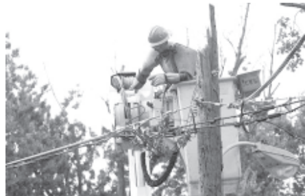
A Pepco contract worker works on a damaged utility pole in Silver Spring, Maryland, on 3 July, 2012. REUTERS
