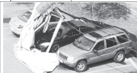
Debris from the storm-damaged Park Tanglewood apartments, some of which were exposed when high winds tore open a hole in the roof and knocked out the electricity, sits atop cars and utility lines in the parking lot in Riverdale, Maryland, 30 June, 2012.—REUTERS
