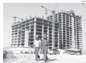
Workers walk in front of a multi-story commercial building under construction on the outskirts of the western Indian city of Ahmedabad on 31 May, 2012.
