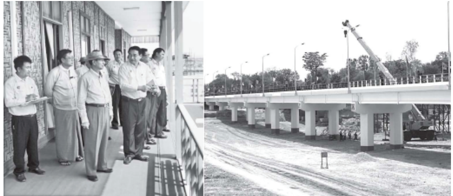
Union Minister for Construction U Khin Maung Myint at bridge construction site.—MNA
