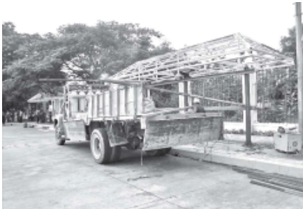
SHELTERS DONATED: Shelter at new Myenigon bus stop in Yangon, donated by private companies, under construction on 23 April.—KYEMON
