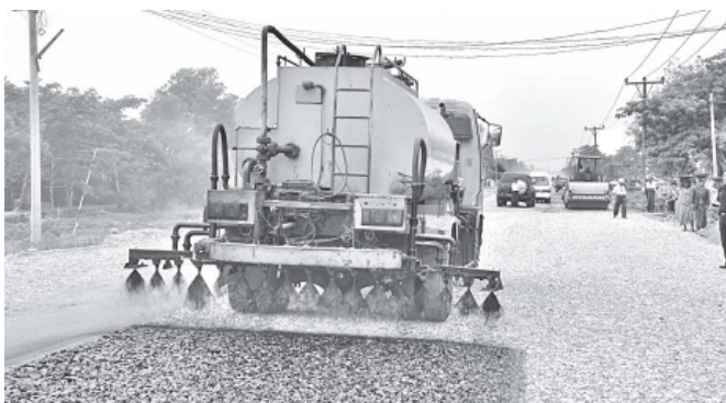
YANGON, 25 May—Upgrading of 22-ft-wide Bohmu Bahtoo road to 48-ft-wide four-lane one is in process. The road is in Dagon Myothit (North). Construction started in
