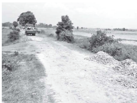
As a gravel road networking from the Kongyi junction on Yangon-Mandalay Pyidaungsu Road to Anauk Uyinhmu Village is beneficial to rural people, Yedash Township Development Affairs Department is now upgrading the road for convenience of the locals.—KYEMON
