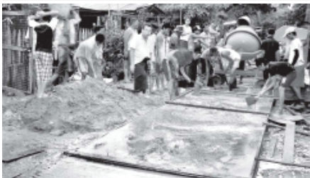
ROAD CONSTRUCTED: Under the supervision of Township Administrator U San Min, local people participate in concreting 4th East Manbye Street on a self-reliant basis in South Ward 2 in Thakayta Township of Yangon Region on 8 May.
