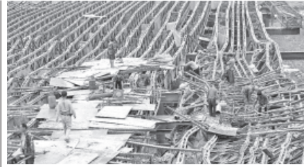
Workers are seen at the dismantlement site of the Lianshuihe Bridge in Loudi, central China's Hunan Province, on 13 May, 2012.—XINHUA
