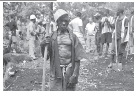
In this 10 April, 2012 photo, Genove Valcimon, 70, poses for a picture as he works on a road being built through the mountains to lead to an exploratory drill site in the department of Trou Du Nord, Haiti. Haiti's land may yet hold the solution to centuries of poverty: there is gold hidden in its hills, and silver and copper too.—INTERNET
