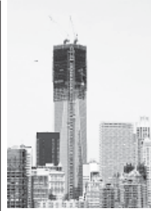
One World Trade Center has become the tallest building in New York City on Monday, overtaking the height of the Empire State Building. The placement of a column of the 100th floor brought the colossal new steel structure of One World Trade Centre tower to a height of 1,271 feet - surpassing the frame of the Empire State Building, which was New York's tallest skyscraper, by 21 feet.—XINHUA
