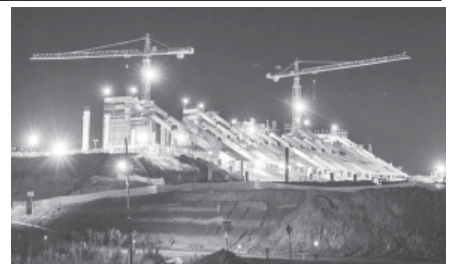
The construction site of a new stadium, Itaquerao, which will be used for the opening match of the 2014 World Cup is illuminated during the night in Sao Paulo on 3 April. Brazil will invest $17 billion on public transport for the 2014 World Cup and the 2016 Summer Olympics, President Dilma Rousseff announced Tuesday.—INTERNET
