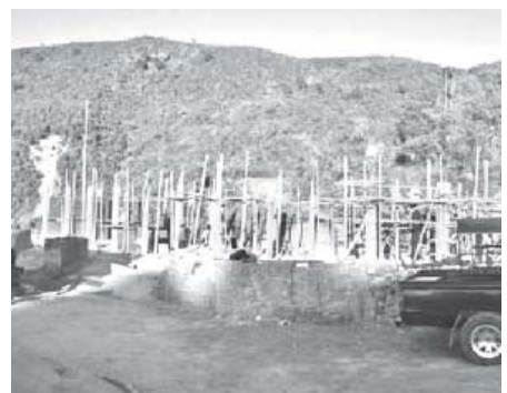
Photo shows progress of construction site for new building of Basic Education Primary School in Thandaunggyi Township.
