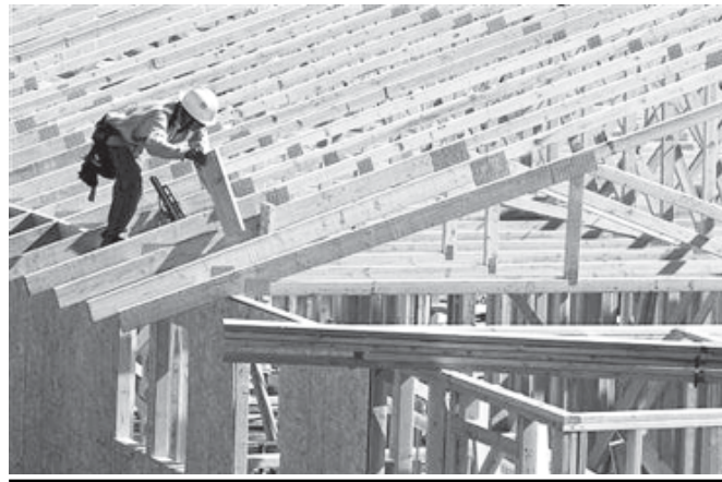
A construction worker builds a new home at a development area in San Marcos, California on 20 March, 2012.—REUTERS
