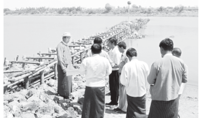
Sagaing Region Chief Minister U Tha Aye inspects anti-bank erosion works at Watchaunglay Village in Kani Township.—MNA
