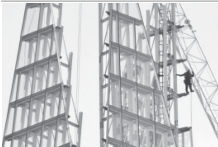
A builder installs glass panels on 1 April, 2012 near the top of the Shard, the European Union's tallest building, in London. The developers building the Shard defended their security measures after it emerged that a group of "urban explorers" had broken into the skyscraper. — INTERNET
