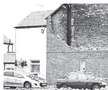
The collapse of a wall at a house which damaged cars in Stoke-on-Trent happened during high winds.
