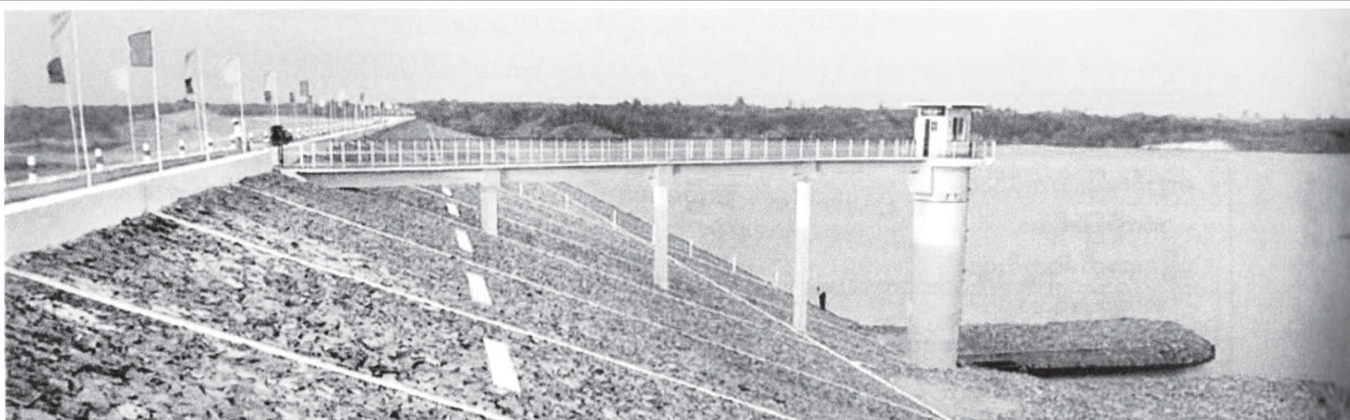
Wahkadok water supporting dam and its control tower.
