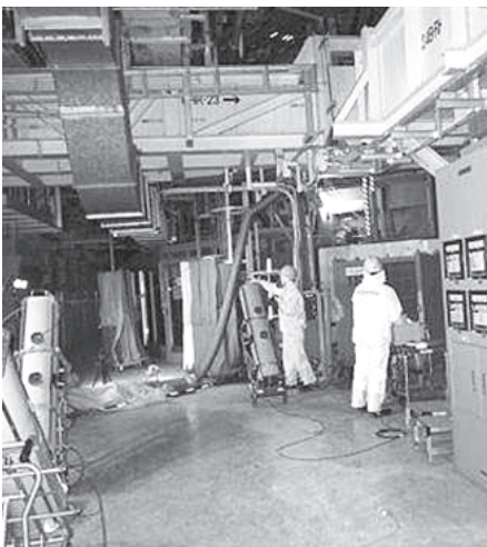
Workers conduct measurements inside the primary containment vessel at Tokyo Electric Power Co (TEPCO)'s tsunami-crippled Fukushima Daiichi nuclear power plant No 2 reactor in Fukushima prefecture, northern Japan, in this handout image taken and released by TEPCO on 27 March, 2012.—INTERNET
