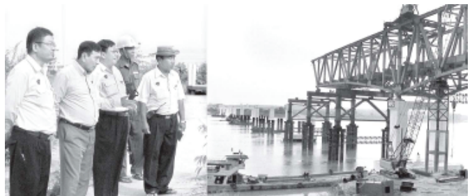
Deputy Minister for Construction U Kyaw Lwin inspects progress in construction of Ayeyawady Bridge (Malun).—MNA
