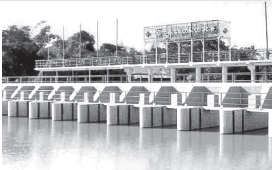
Seikkyun Sluice Gate near Seikkyun Village in Thaton Township, Thaton District, Mon State, supplying water for growing monsoon and summer paddy.
