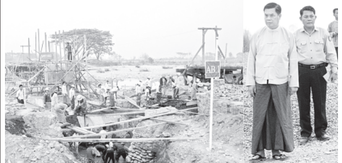
Sagaing Region Chief Minister U Tha Aye inspects construction of Nattaga Creek Bridge in PyindawU Village of Kalay Township.
