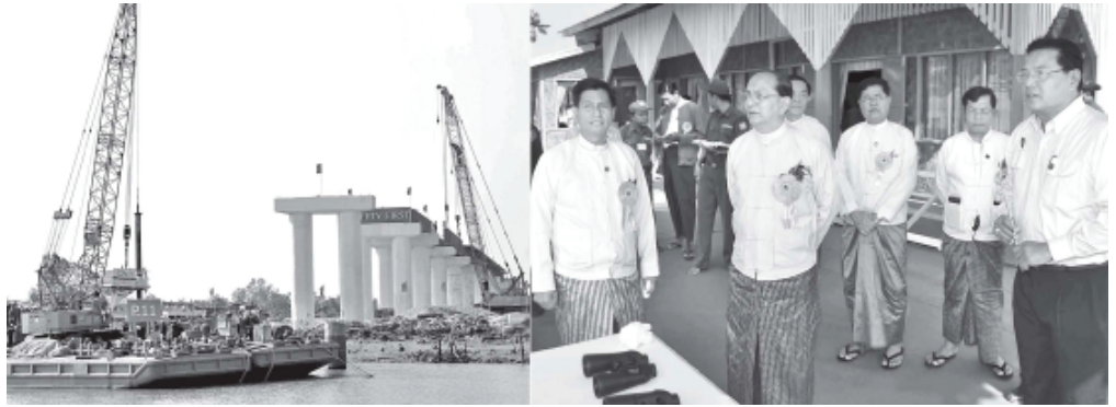
President U Thein Sein inspects progress in construction of Thetkel Creek Bridge.—MNA
