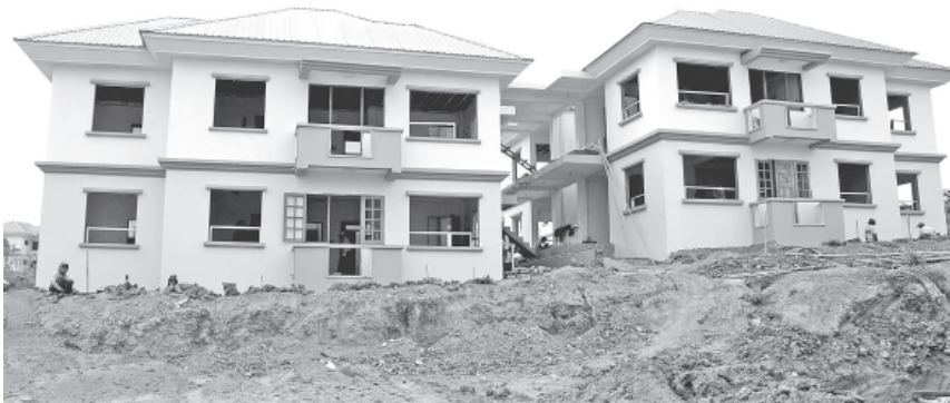
Lodgings for sport athletes under construction at Sports Village Project in Nay Pyi Taw.—MNA
