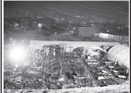
Firefighters and police attend the scene of a fire at a construction site in the Esenyurt district in Istanbul. INTERNET
